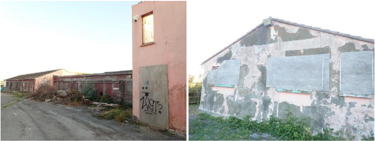
External photographs of western building: Eastern elevation (left) and (right) southern elevation with boarded up windows.
