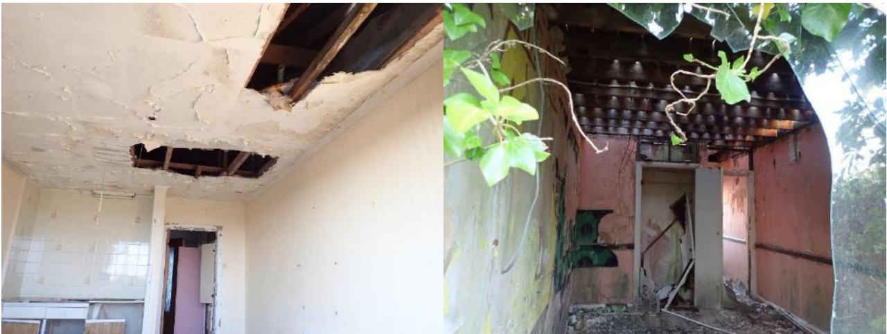
Internal photographs of western building: Missing ceiling plasterboard (left) and (right) exposed joists and broken window.
