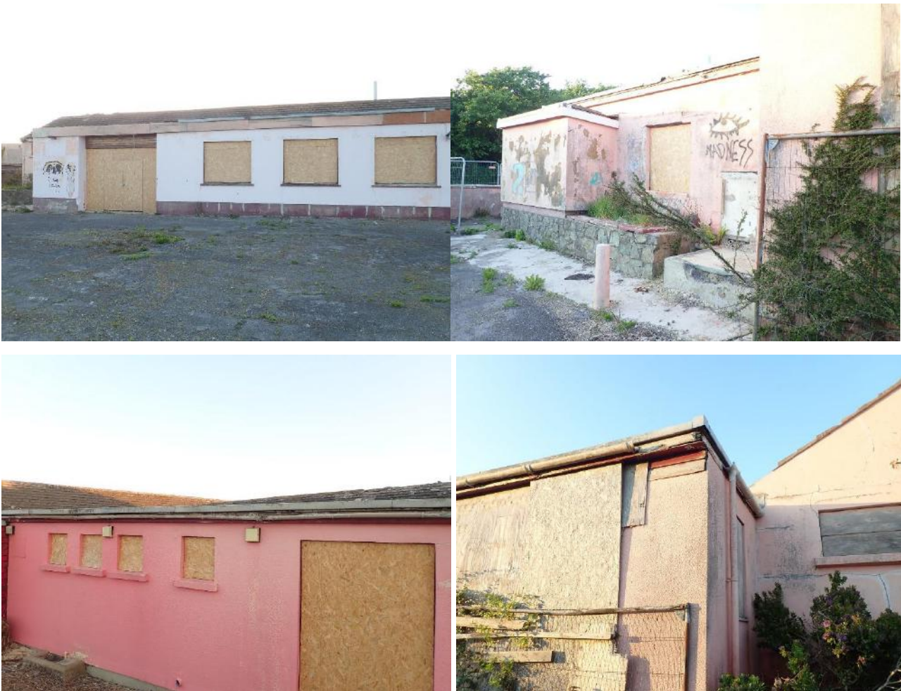
External photographs of eastern building (Clockwise from top left): Southern elevation with boarded up windows and doors, and mainly intact roof; western elevation with flat roof; potential squeeze gaps behind boarding and at corner of soffits; eastern elevation.
