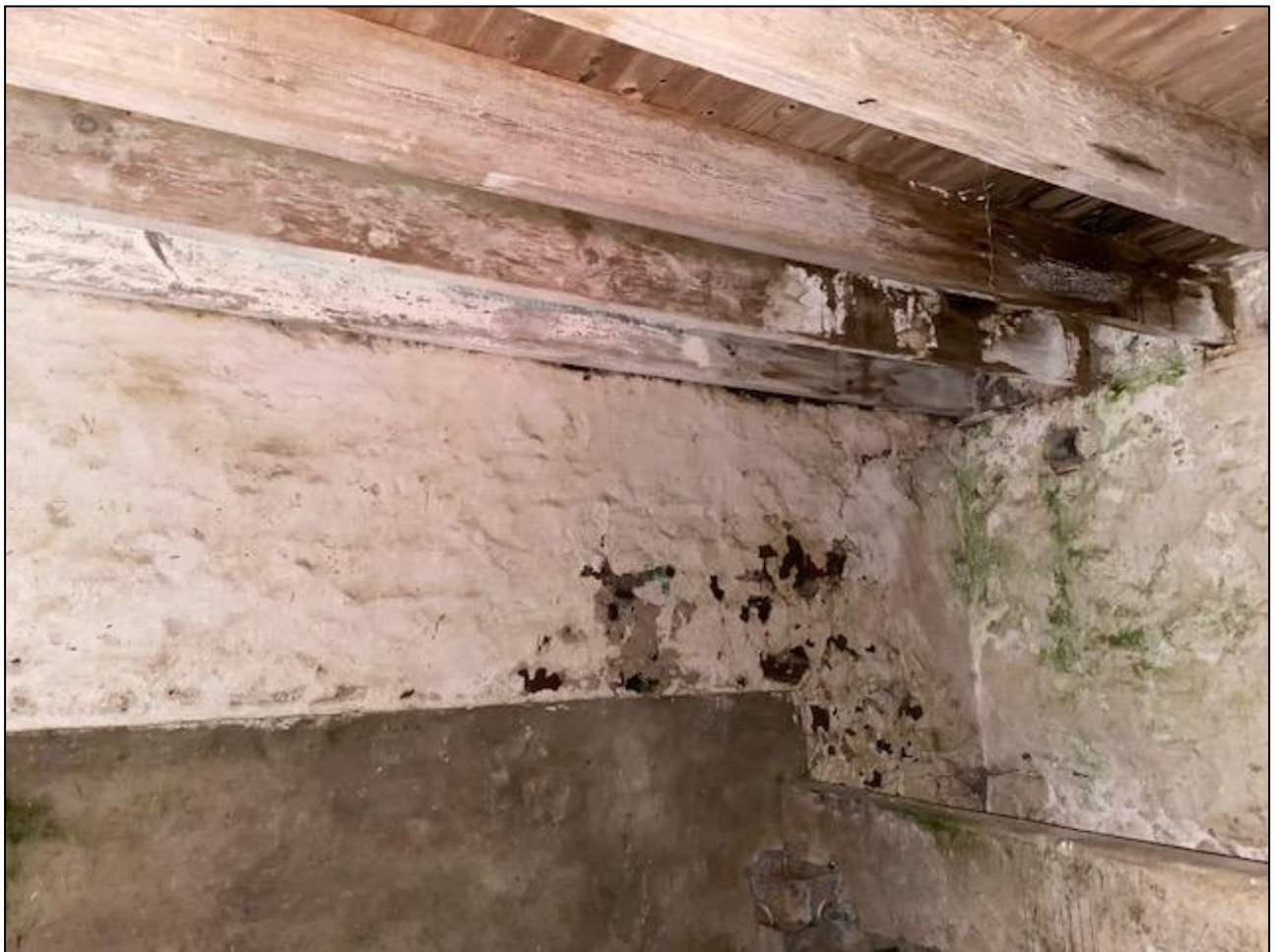
Figure 5. Gap between wall and floor used by three brown long eared bats on north western gable end wall.
